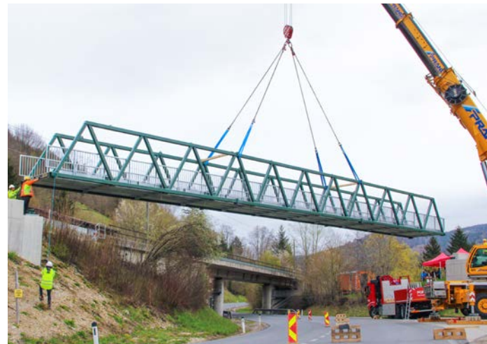
Successful lift to close the gap of the superregional R16 cycling track.
