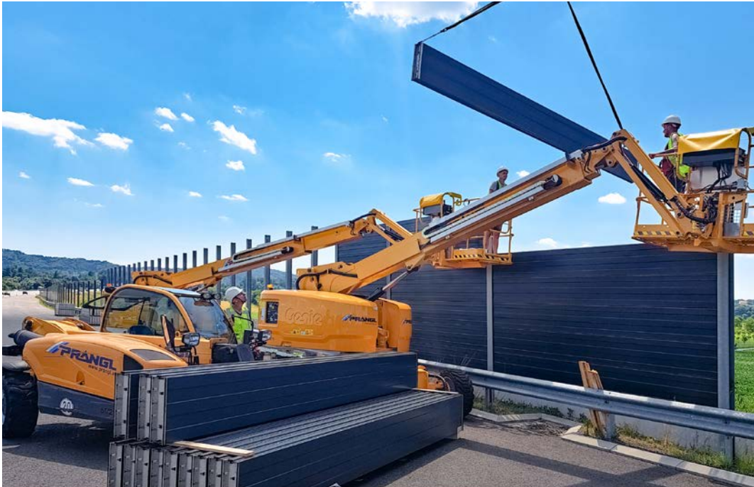
Fitters at work: Forster was also commissioned with supplying and installing the noise protection systems.
