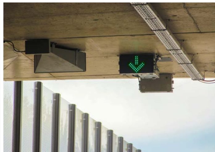
Twenty-four continuous light signs indicate the open and closed lanes in the tunnel.
